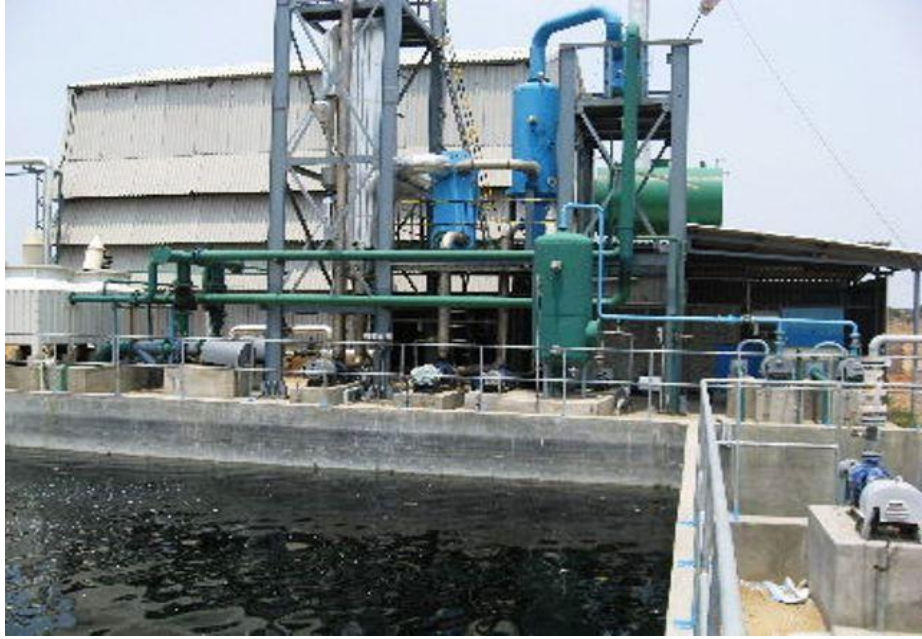
Zero Liquid Discharge System
