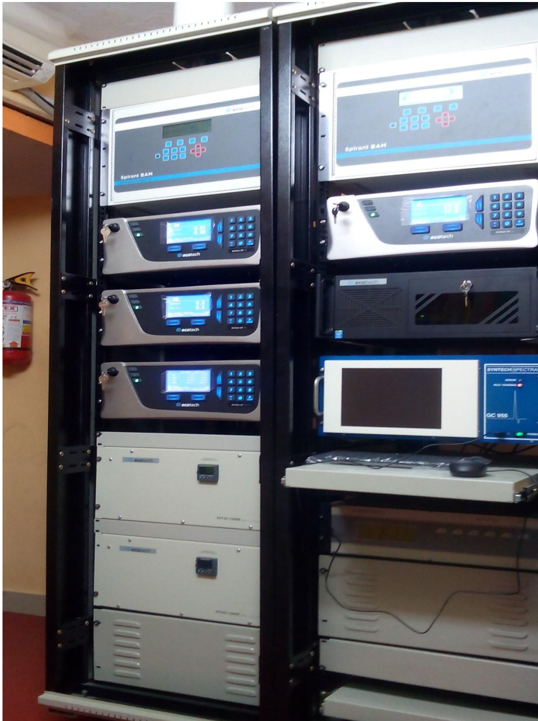
Continuous Air Monitoring At Perungudi
