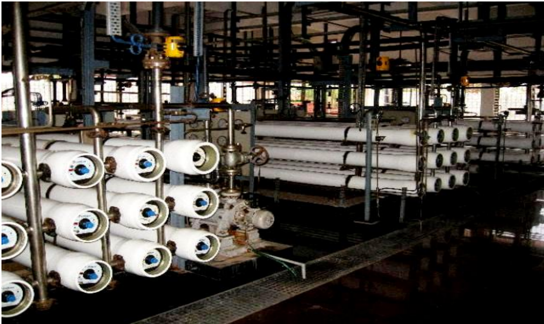
Reverse Osmosis Plant
