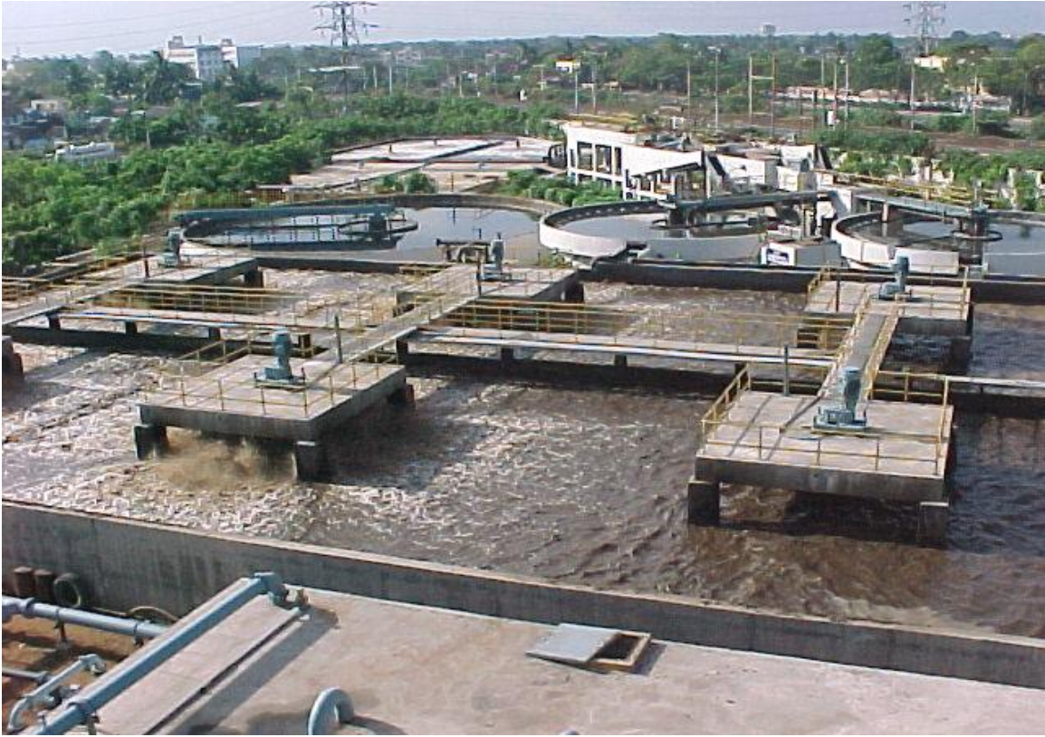
Sewage Treatment Plant in Thermal Power Station
