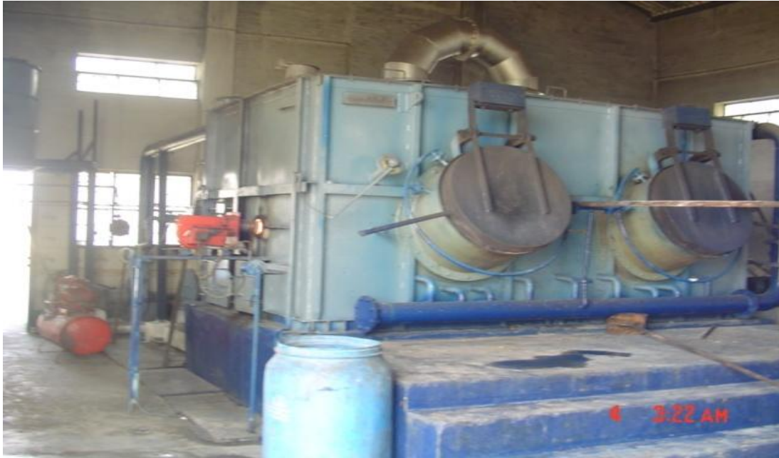
Common Bio Medical waste Incinerator
